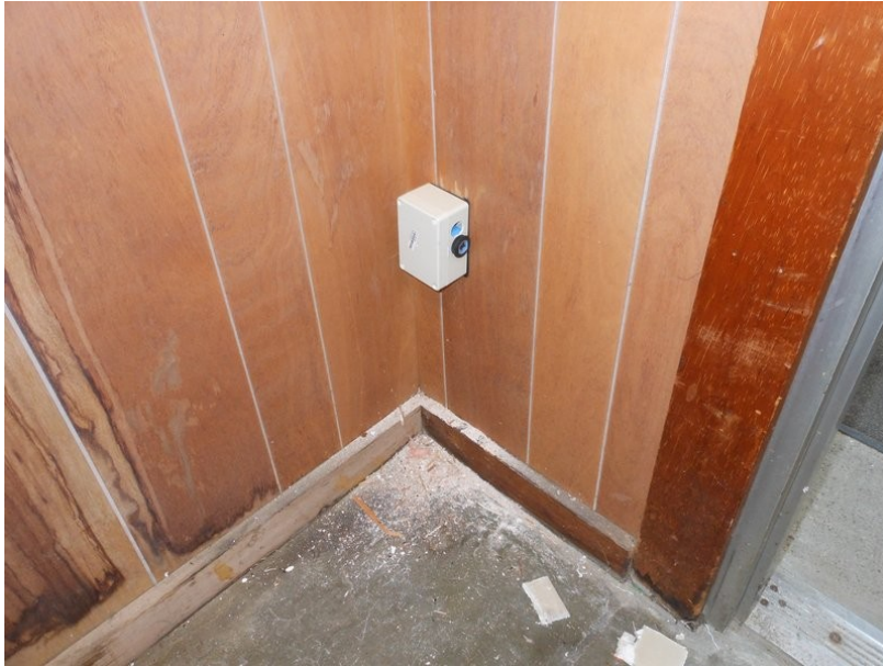
Box installed on the wall. This is a temporary box I used for testing purposes. The additional hole at the top is an error, but allows viewing the LED (though this sensor does not change its LED colour, it's always green).
