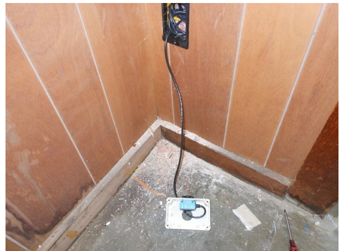
Installing the single sensor. I used ethernet as the power line. I also used a passive PoE adapter on both sides to transfer the power onto the ethernet, and back out to a 5.5, 2.1mm barrel plug
