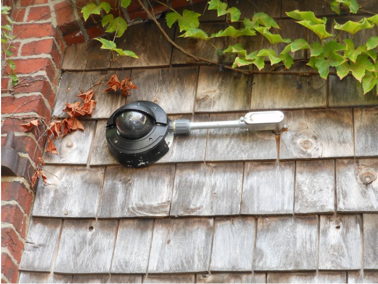
Figure 5: After: Camera is installed.
