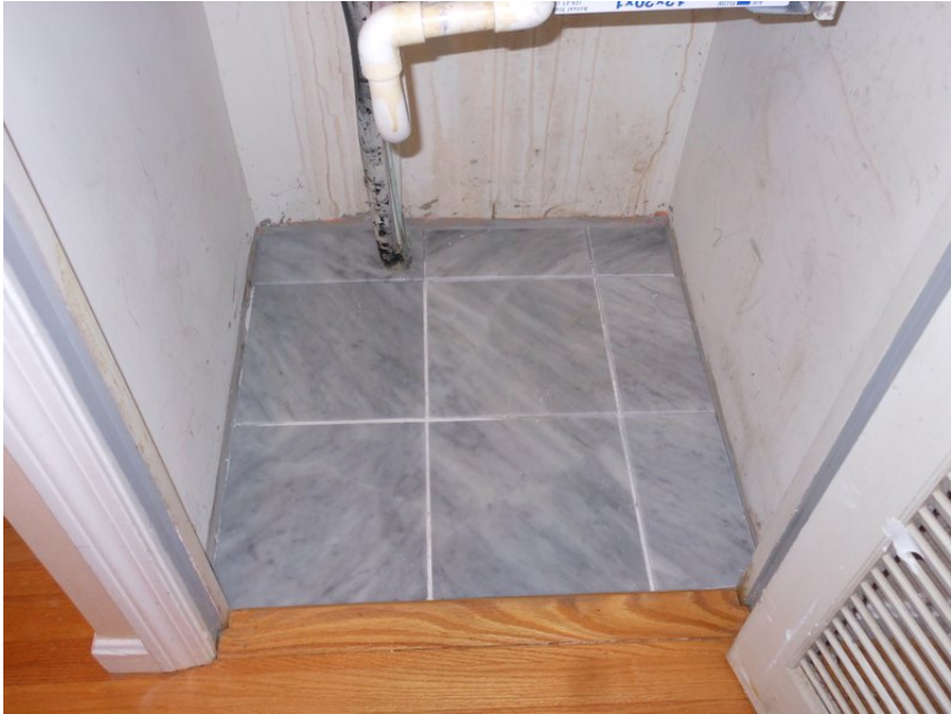
Figure 2: After. In this picture, the back tiles, and the right side are cut, but not actually in mortar. This is just to get a look at how it should appear. Tiles are cut in day five.
