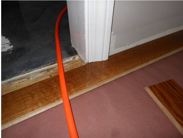
Figure 4: Hardwood fitting underneath the door trim. Wall trim has been removed until the floor is in place.
