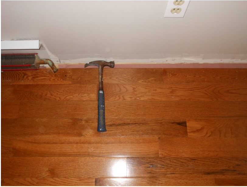
Figure 11: When getting to the opposite wall, a hammer can be used to pry or push the wood towards itself. With a buffer piece of wood when possible. Here the pneumatic finishing gun is used, and not the hardwood nailer, as it can't fit. Without the hardwood nailer, it gets difficult to compress these particular planks, so some creative type of spreader was needed. Higher grade hardwood might be easier to use.
