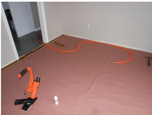
Figure 1: Here the pink Rosin paper has been placed down in sheets, and the first row is being started. Hardwood nailer in foreground.
