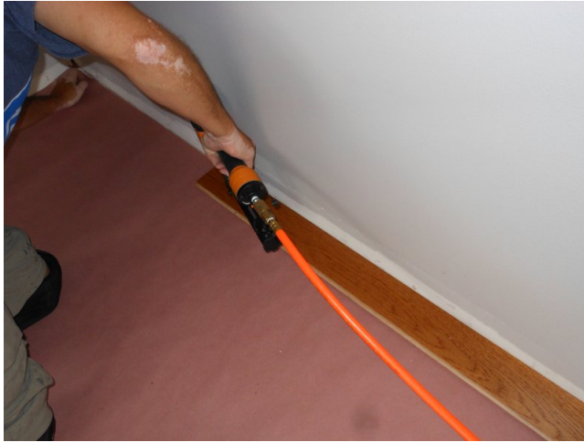
Figure 5: Pneumatic (not hardwood) Nailer used for first or second row, because the hardwood nailer won't fit. Nails are put on top of wood. Later, the mallet-powered hardwood nailer will put nails on the edge of the wood at an angle, so they are invisible.
