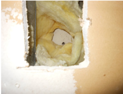
Figure 2: This hole went above the drop ceiling, through the old and new drywall, and also some insulation.
