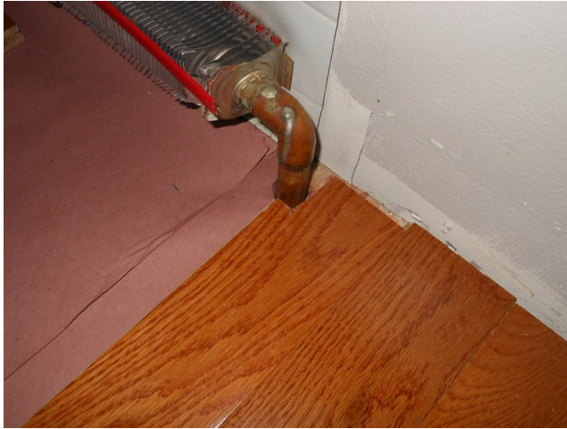
Figure 7: Cuts are made around hot water heater pipes. Beware of cracking the pipes when working around them. This particular heater pipe has a cover, so this cut did not necessarily need to be precise.
