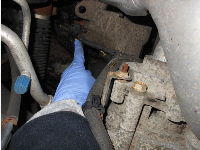
Figure 2: Wires visibly chewed here
