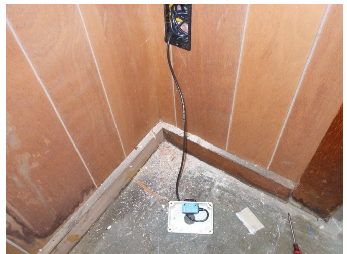
Installing the single sensor. I used ethernet as the power line. I also used a passive PoE adapter on both sides to transfer the power onto the ethernet, and back out to a 5.5, 2.1mm barrel plug
