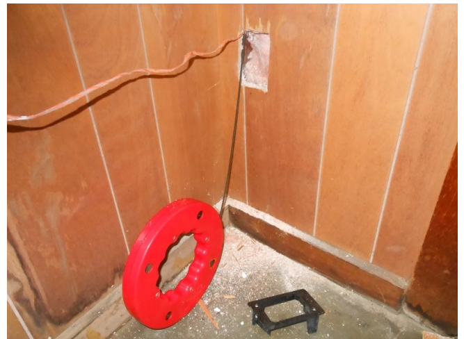
Feeding nylon string, and a wire up from the bottom of the wall to the ceiling. This is where the
