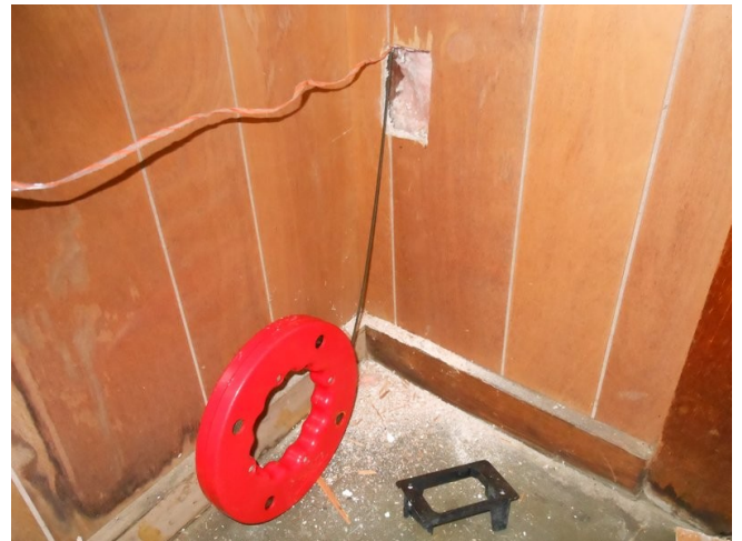
Feeding nylon string, and a wire up from the bottom of the wall to the ceiling. This is where the single sensor will be.
